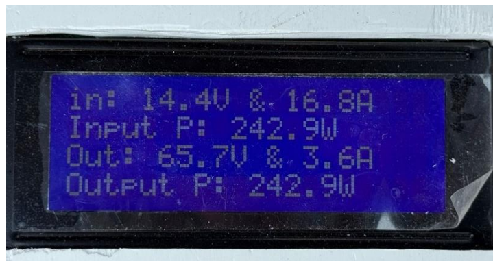
Figure 4.10: LED Display (MPPT Charge Controller Output)
